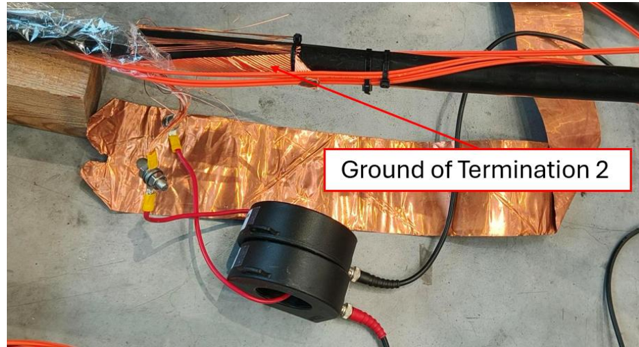
Second termination ground with HFCT50 connection
